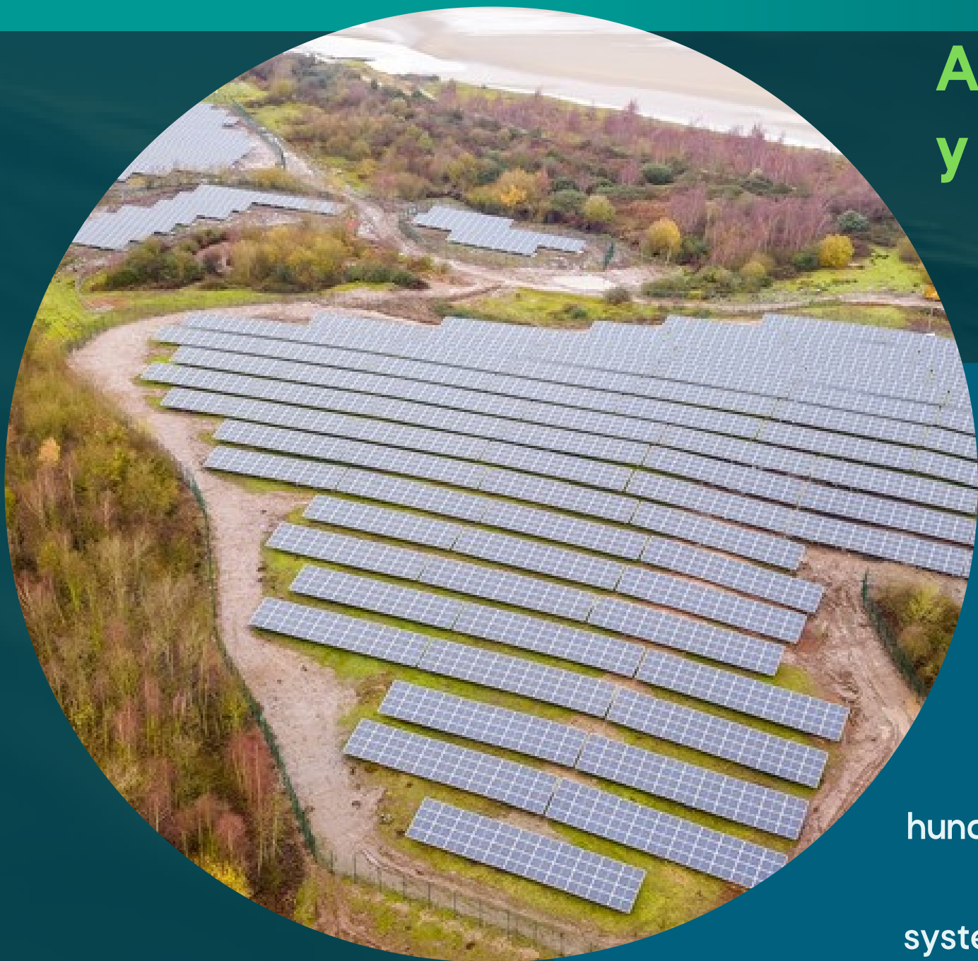
Ffigwr 05: Crumps Yard, Cei Connah Llun: © SMA Solar Technology UK Ltd (Fferm Solar Sir y Fflint)
